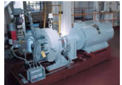
150 kW back-pressure turbine generator installed at the district heating plant of the Franciscan Sisters of Perpetual Adoration in LaCrosse, Wisconsin, USA.
